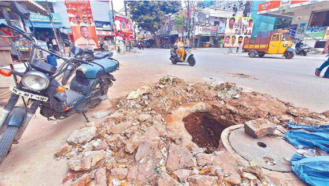
A large manhole has emerged after a newly laid road was damaged at Shalivahana Nagar, behind Dilsukhnagar Bus Depot, posing a serious risk to motorists and pedestrians Photo: Srinivas Setty
