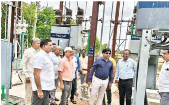
APSPDCL CMD Siva Sankar Lotheti inspecting substation in Pileru division on Friday
