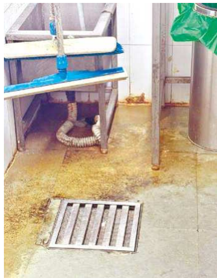
Unhygienic kitchen conditions observed during Food Safety Department inspections at food establishments
