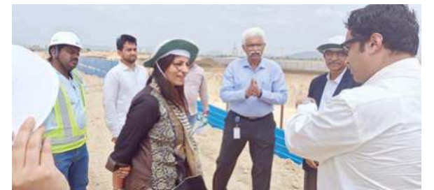
Gates Foundation India Country Director Archana Vyas at the construction site of the upcoming Basavatarakam Indo American Cancer Hospital at Thullur in Amaravati on Friday
