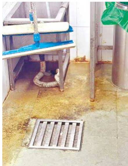
Unhygienic kitchen conditions observed during Food Safety Department inspections at food establishments
