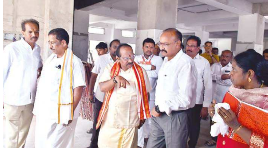
Endowments Commissioner K Ramachandra Mohan, Sri Durga Malleswara Swamy Varla Devasthanam Trust Board Chairman Borra Radhakrishna (Gandhi), and senior officials inspecting the ongoing construction works of the new Laddu Potu and Annadanam Complex at the Kanaka Durga Temple atop Indrakeeladri on Thursday
