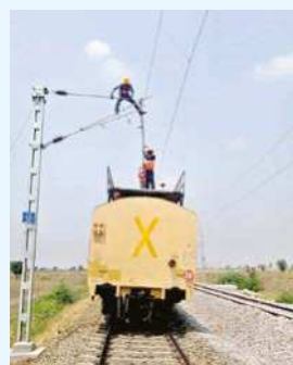
3.05 am on Thursday between Tehta and Jehanabad stations in the Gaya-Patna section, disrupting train services. Affected down trains were operated under single-line working. The electrical wire was repaired by railway staff and declared fit at 6.26 am, the CPRO added.
