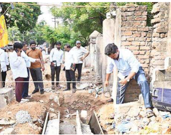
Municipal Commissioner YO Nandan inspecting drainage canal works in Nellore on Wednesday
