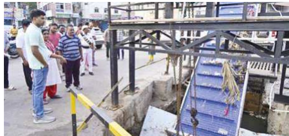
VMC Commissioner HM Dhyanaachandra inspecting the ongoing desilting works at Krishnaveni Cloth Market on Tuesday
