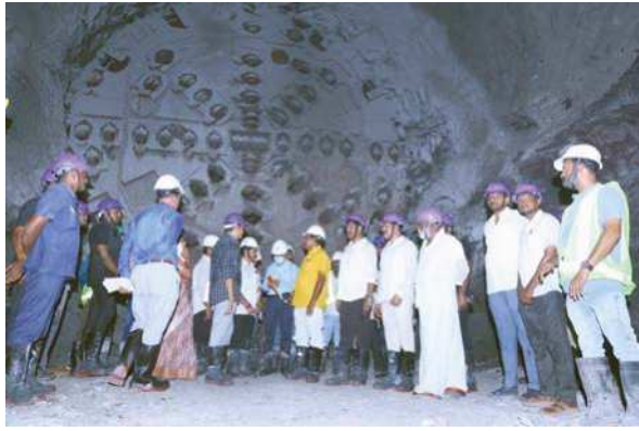
Minister Nimmala Rama Naidu, MLA Kandula Narayana Reddy and others inspecting Tunnel Boring Machine in the tunnel of Veligonda Project on Tuesday
