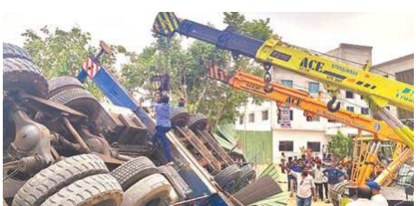
An overturned crane and rescue machinery at the hotel construction site on DBR Road in Tirupati. The fatal accident claimed three lives
