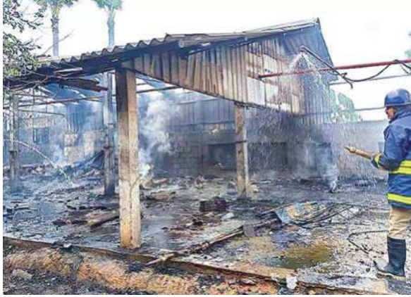
Aftermath of the blaze in Grand Fireworks at Rayavaram village of Dr BR Ambedkar Konaseema district last October
