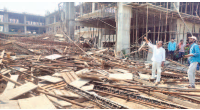
Construction site where centring collapsed in Mahabubabad on Monday
