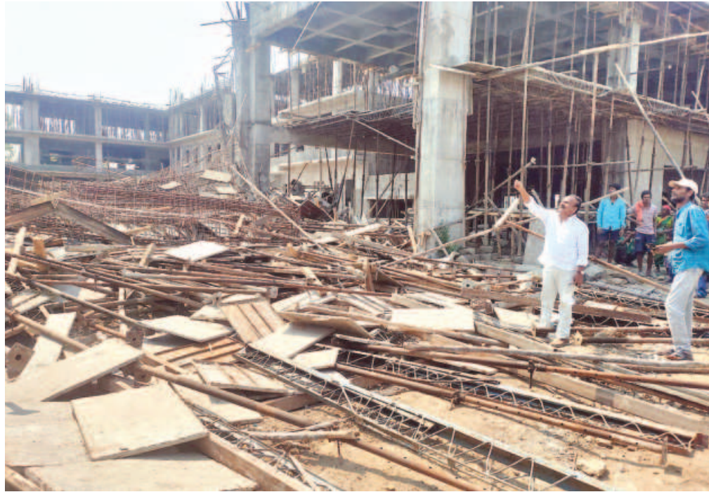
Construction site where centring collapsed in Mahabubabad on Monday
