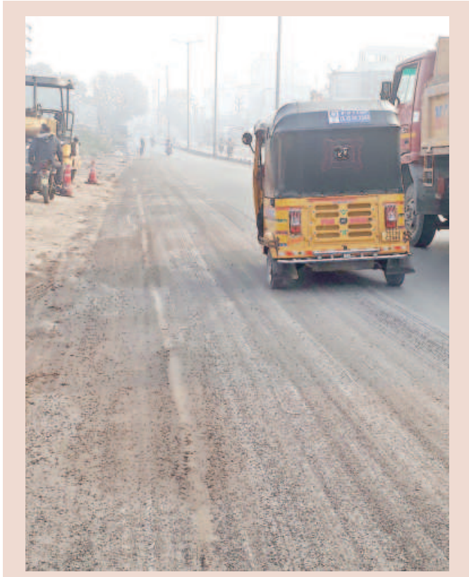
Road works are being taken up under Comprehensive Road Maintenance Programme (CRMP) in Rajendranagar
